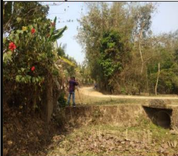
3. RCC culvert to carry excess rain water
